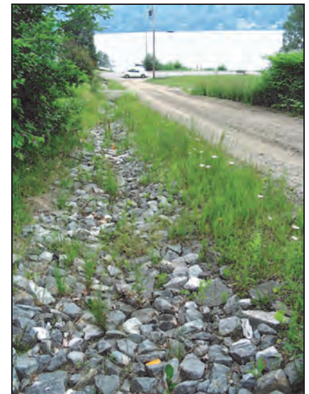
A steep road that serves several camps with a rock lining installed to prevent the previous on-going erosion of the ditch.
